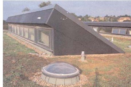
The grass roof provides thermal mass and insulation for the school, while the clerestory windows provide daylight and ventilation (above)
